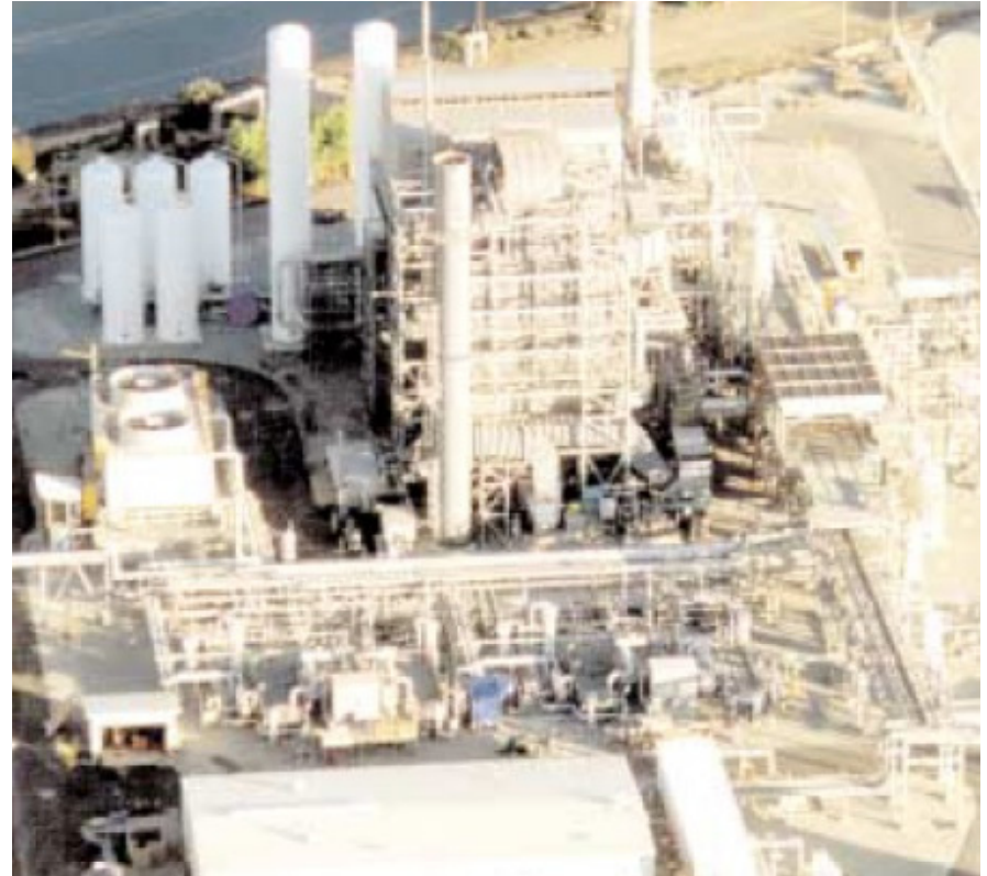
Air Products 96 MMSCFD SMR in Carson, CA is connected to a pipeline with another Air Products SMR, allowing refineries to meet environmental regulations and enjoy benchmark reliability.
