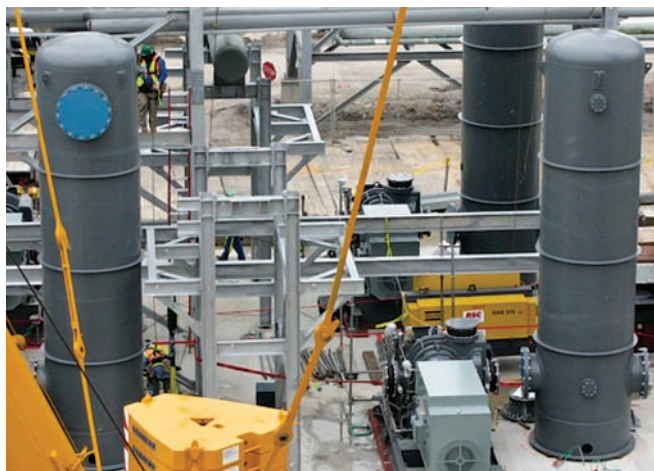
FIG. 5. VSA vacuum blowers are used to recover CO 2 from the VSA beds and deliver it to the CO 2 product compressor before offsite transport via pipeline for use in EOR.
